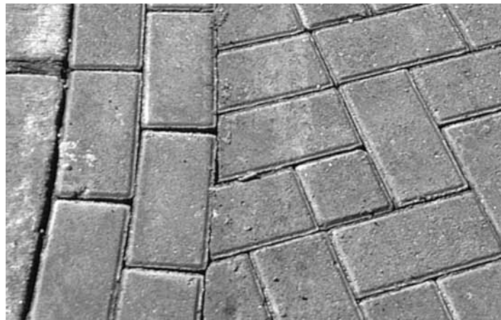
Figure 14. A double row of manually placed pavers along a curb or building provides maneuvering space for the mechanical installation clamp.
