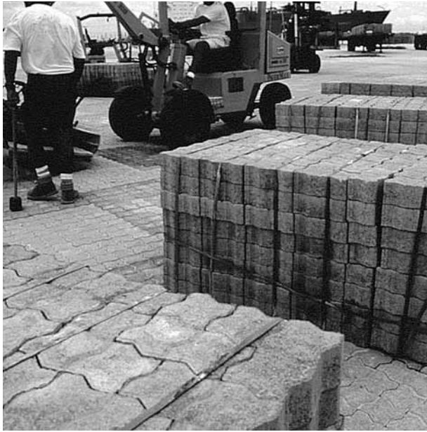
Figure 15. Spacing of cubes at the laying face is determined by how much area will be covered by each, as well as by the clearance required by the machine clamp. Orientation of the cubes follows the direction of paving.
