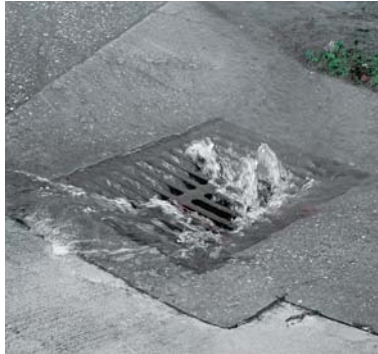
Stormwater Inlet Drain - Lake Park, FL
