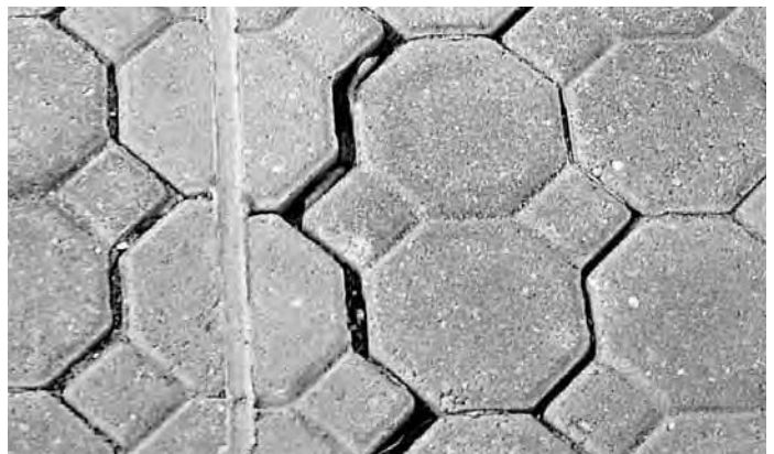
Figure 12. An absence of edge restraints and use of a sealant in this construction joint caused the pavers to shift and open their joints on both sides of the sealant.
