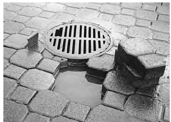
Figure 15. An absence of holes in the sides of this roof drain led to ponding.
