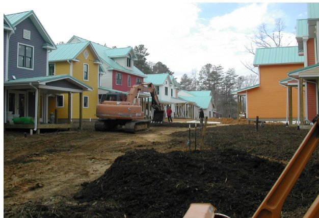
Figure 6-3a and b. Debris and stump grinding at the Pacifica (North Carolina) LID project (top); spreading of stumps ground for mulch (bottom)
