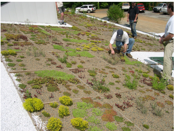
Figure 8-22. Green roof at the North Carolina Arboretum Operations Center during routine maintenance
