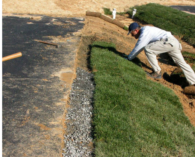
Figure 4-16. Installing a gravel verge and sod stabilizes the perimeter of bioretention cells and is highly recommended. The resulting filter strip shown here is nominally 5 feet wide.
