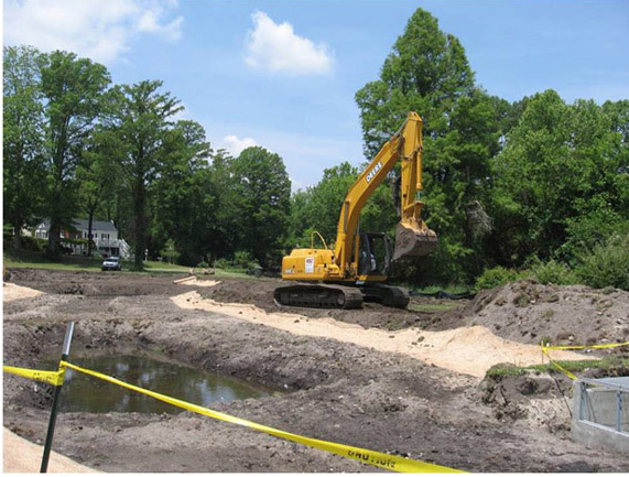
Figure 7-9. Erosion control fencing protects a creek during construction of a wetland in Wilmington, North Carolina
