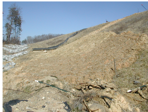
Figure 6-4. Dredged sediment dumped next to the sediment trap with no vegetation or cover
