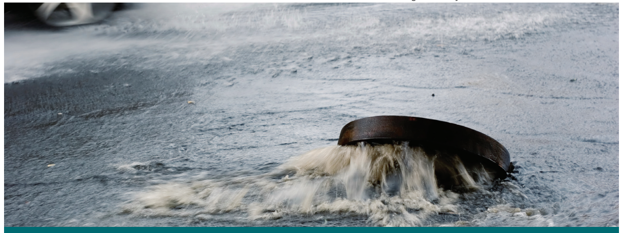
Figure 1.4.1: Even new municipal stormwater infrastructure can fail during extreme weather events.
