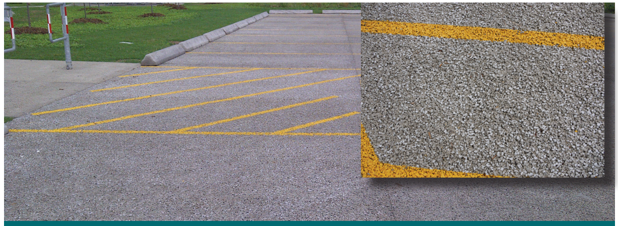
Figure 2.3.1: Pervious concrete and other permeable materials are ideal for overflow parking lots, such as this one constructed at Lakeside Park in Mississauga. (Source: Aquafor Beech)
