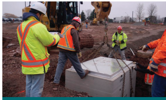
Figure 2.6.5: To maximize treatment benefits, proprietary stormwater treatment devices can be installed upstream of LID practices. For instance, when retrofitting their parking lot, the IMAX Corporation had a proprietary treatment device installed to provide pre-treatment for a bioretention practice. The use of these two practices in series ensured that only the highest quality water would leave their site and be discharged to the environmentally-sensitive Rattray Marsh. (Source: CVC)
