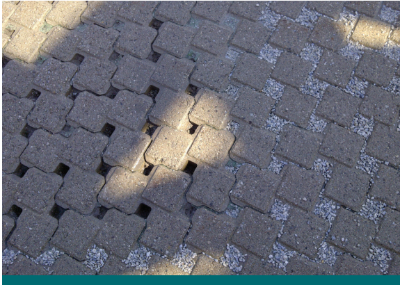
Figure 8.3.1: In this photo the aggregate has been removed from permeable interlocking concrete pavers. This will need to be replenished immediately to avoid clogging of the joints. (Source: Aquafor Beech)
