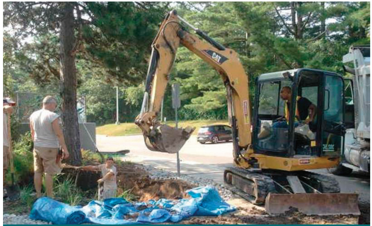
Figure 7.4.1: At Green Glade Sr. Public School, the bioretention soil media originally supplied did not meet the specifications. Due to an improper mixing process, the content of fines was too high. To rectify the problem, the soil was removed and replaced with the specified bioretention soil media. (Source: CVC)
