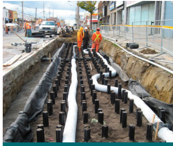
Figure 2.6.2: Installation of soil support system underneath the sidewalk on part of The Queensway, in Etobicoke. (Source: Deep Root Inc.)
