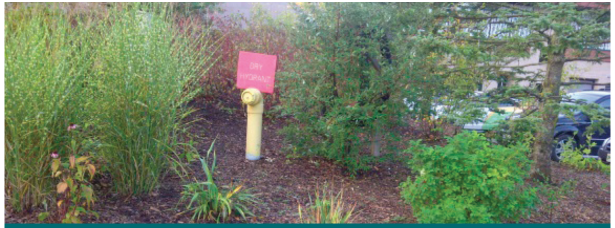
Figure 4.3.2: This dry hydrant is connected to a large subsurface cistern. This water supply can be used in emergency situations to fight fires on site. (Source: Aquafor Beech)
