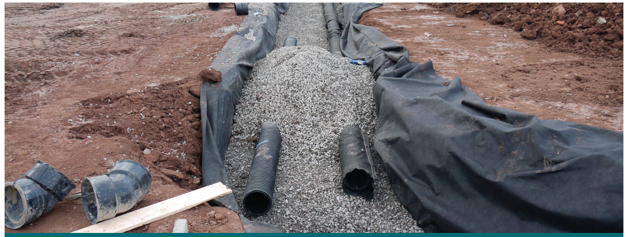
Figure 3.1.2: Permeable pavement and bioswales are being constructed in this parking lot. This requires complete removal of the existing asphalt and granular bedding. Consider a parking lot retrofit when this type of area needs major rehabilitation. (Source: CVC)
