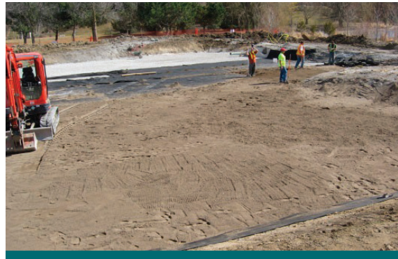
Figure 2.6.4: Installation of a red sand phosphorus filter system during the retrofit of George Richardson Stormwater Management Pond in Newmarket. See the case study in Appendix B for further details. (Source: LSRCA)
