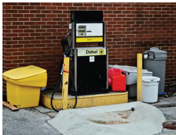
Figure 2.10.2: A fuel pump spill containment pad is recommended for all sites. In case of a spill fuel is detained within the pad until safe disposal. (Source: CVC)
