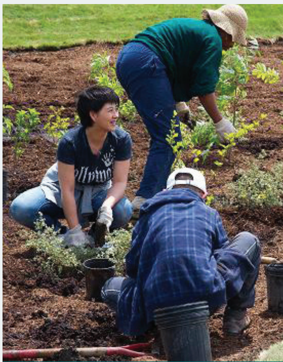
Figure 1.8.2: To help keep costs low, volunteers helped with construction of a rain garden at Portico Church in Mississauga. The project received funding from Walmart-Evergreen Community Grants and Sobey's Community Environment Fund. (Source: CVC)
