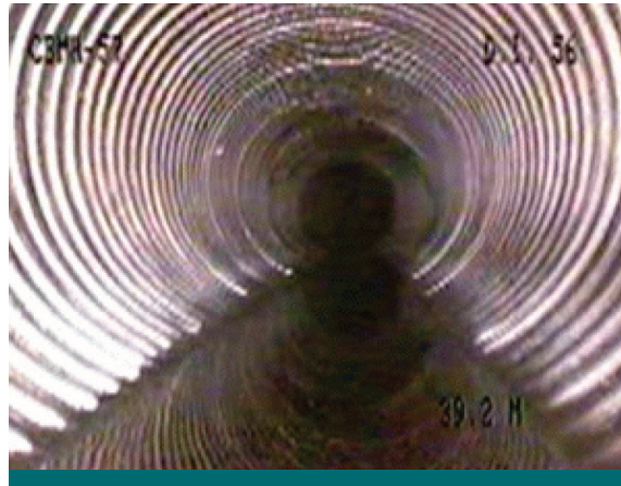
Figure 8.2.1: Video inspection (pipe scoping) is a rapid means of identifying any issues with buried pipe. Look for any indications of pipe collapse, blockages, or sediment build-up. This photograph from an Ottawa perforated pipe shows it to be in excellent condition even after more than 20 years of performance. (Source: City of Ottawa)
