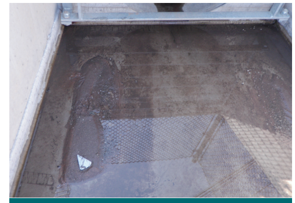
Figure 8.4.2: Along with measuring sediment depth in a proprietary stormwater treatment device, check the outlet structure (if accessible). If the device was functioning as intended this sedimentation should not be occurring, unlike in the device pictured. (Source: Aquafor Beech)
