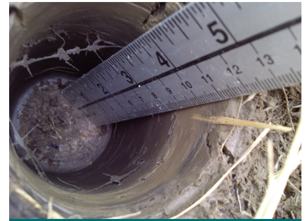
Figure 8.1.2: At this site, coring indicates a layer of impermeable clay has clogged this bioretention unit. Major rehabilitation including replacement of the bioretention soil media will be required for proper filtration and infiltration. (Source: Aquafor Beech)
