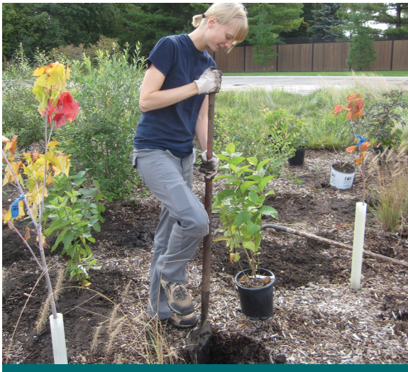
Figure 6.2.1: In this photo, a volunteer from a local conservation authority helps with planting a church's new parking lot bioretention cell. There are many organizations that can help you understand how to maintain an LID feature. (Source: CVC)
