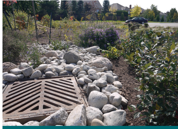
Figure 6.3.3: At PORTICO Church green areas adjacent to the parking lot were targeted for bioretention practices. (Source: CVC)
