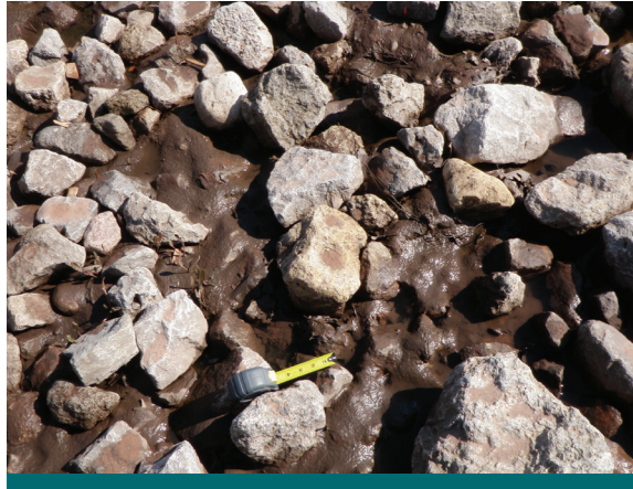
Figure 8.1.1: Closely inspect any pre-treatment areas for excessive sediment accumulation from exposed soil during construction. In this photo a riprap spillway between the forebay and bioretention facility has been subject to clay deposition from upstream construction. (Source: Aquafor Beech)
