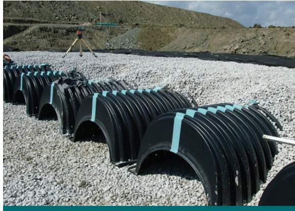
Figure 6.3.2: Infiltration chambers are often buried below parking lots. This photograph shows how they look before they are covered over during construction. (Source: Aquafor Beech)
