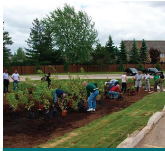
Figure 6.2.2: Faith-based youth groups may be another source of volunteers for your retrofit. (Source: CVC)
