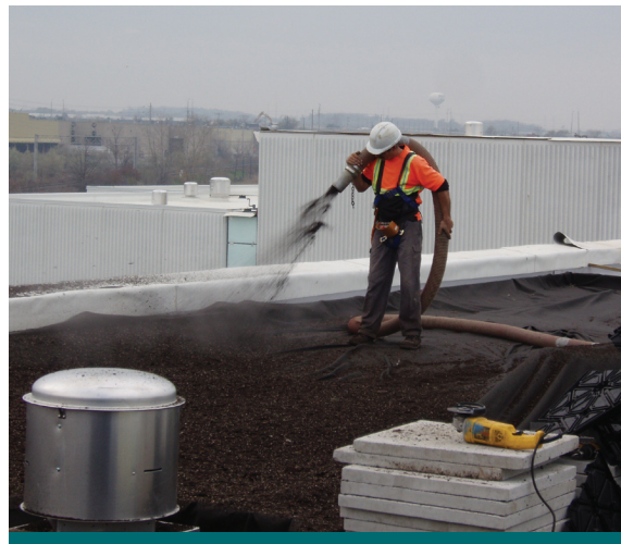
Figure 2.9.1: Green roofs must be designed and constructed around structural, drainage, ventilation and mechanical components. (Source: CVC)
