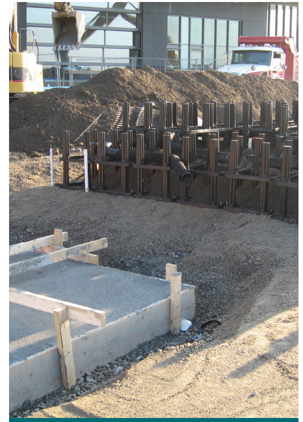
Figure 4.4.4: At this site, a soil support retrofit is being integrated with the replacement of an adjacent parking lot. Sharing resources to complete two retrofits at the same time can save on costs (Source: Deep Root)
