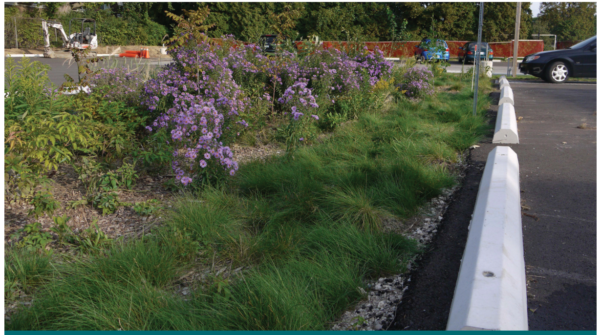
Figure 6.1.1: The Unitarian Church in Mississauga installed this bioretention feature as part of a parking lot retrofit. (Source: CVC)
